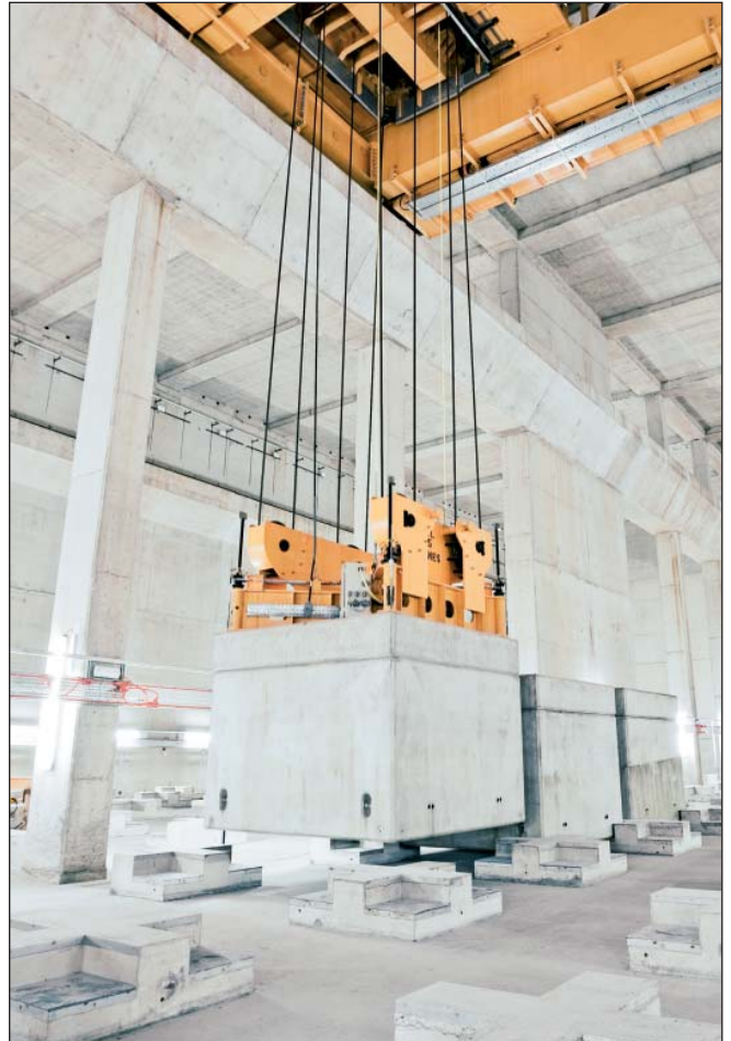
Inside the ILW Store at Trawsfynydd
