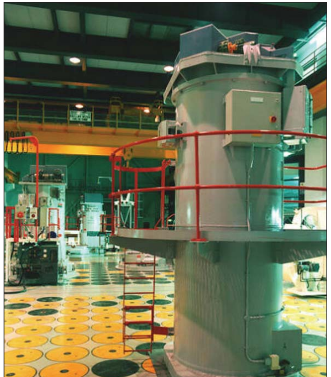
Store for packaged HLW canisters
